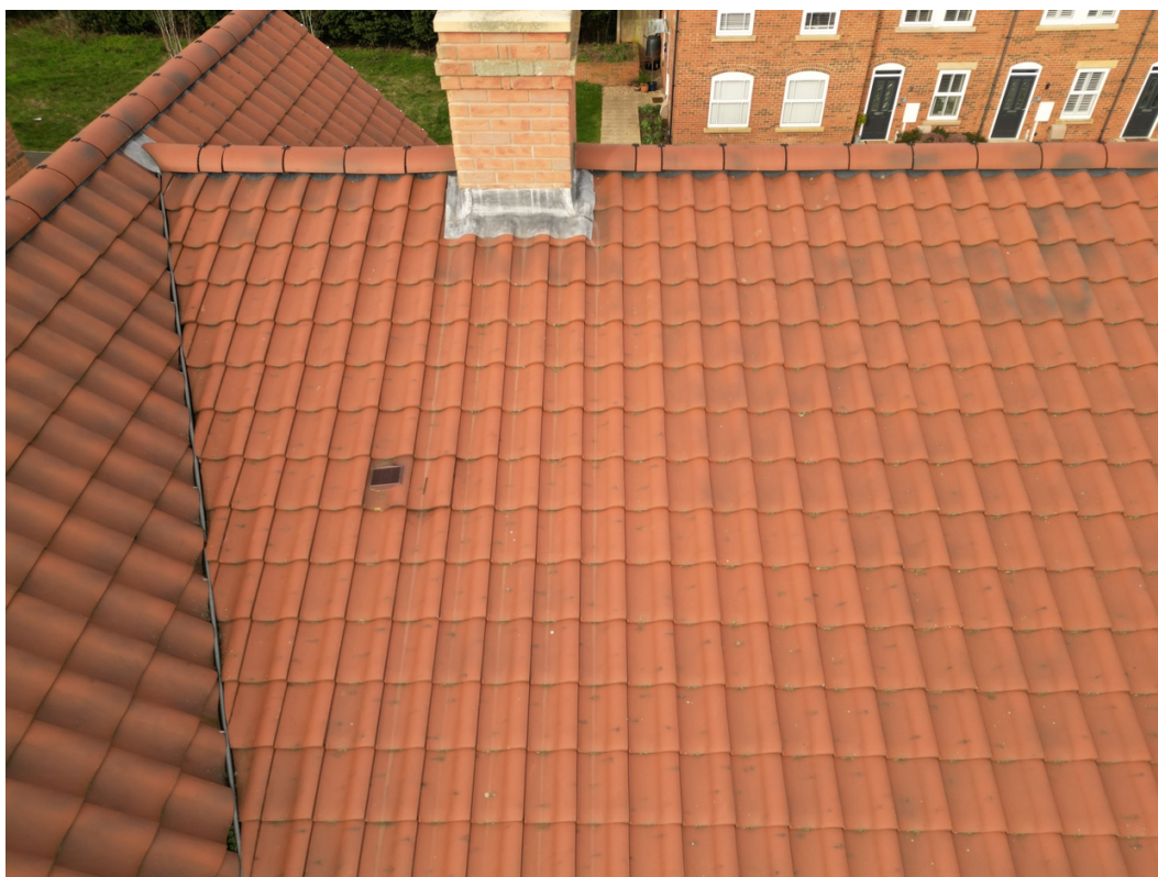
Fig. 3 — Oblique aerial view of the main roof slope showing the chimney stack and roof vent tile (visible below and to the left of the chimney). The vent tile sits within the main field of interlocking tiles on the principal roof slope.
