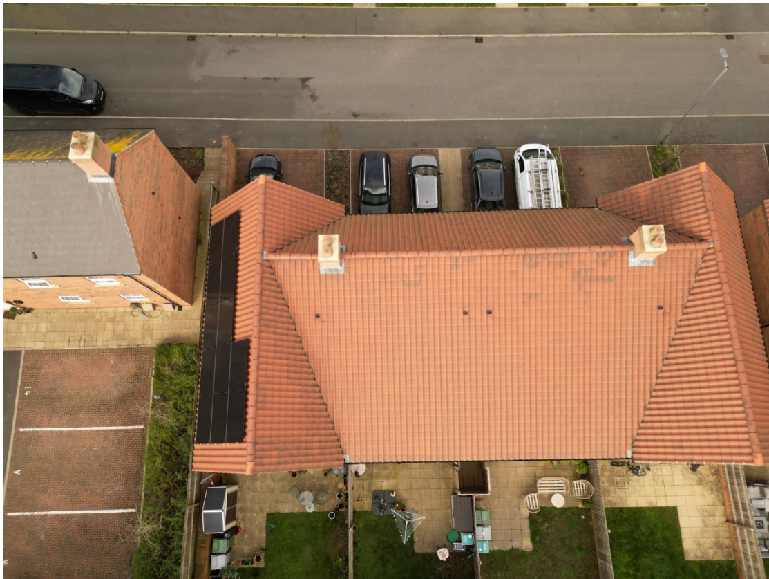
Fig. 1 — Top-down aerial view of the full roof area. Clay interlocking pantiles in generally sound condition. Two chimney stacks visible with lead flashings intact. Roof vent tiles visible on the main roof slope. Solar PV panels on the adjacent property (left).
