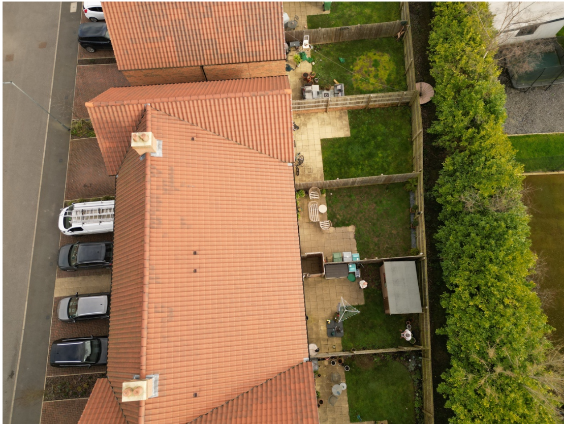
Fig. 2 — Top-down aerial view from alternative angle showing the full roof and surrounding context. No visible signs of widespread tile displacement, delamination, or structural movement. Ridge line and hip junctions appear true and correctly aligned.
