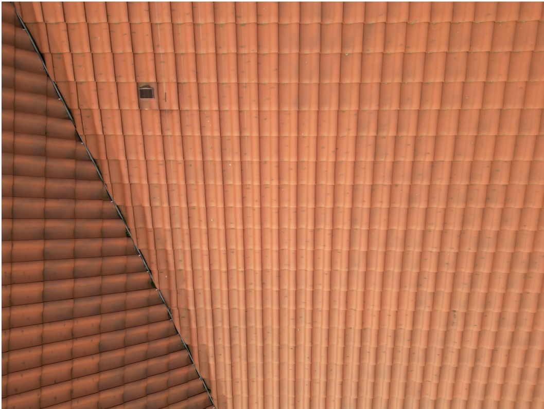
Fig. 4 — Close-up aerial view showing the interlocking tile profile and vent tile position. The tile trough (low channel between profiles) can be clearly seen running directly into the vent location, confirming the water channelling effect described above.
