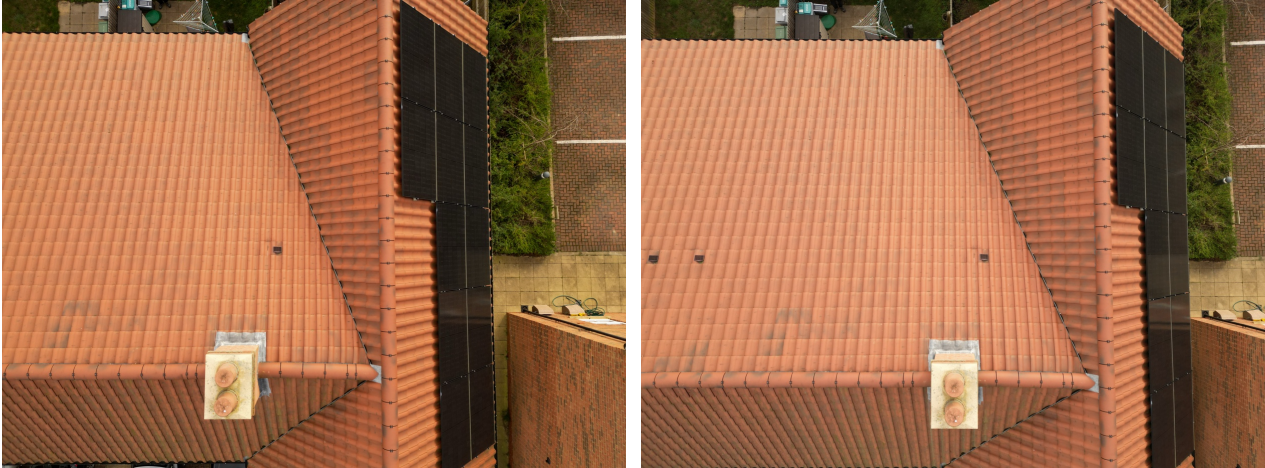
Fig. 5 & 6 — Chimney stack detail showing twin clay pots, lead flashing apron, and stepped/back-gutter flashings. Solar PV panels visible on the adjacent building's roof slope. The chimney flashings appear to be in serviceable condition with no obvious lifting, cracking, or separation at the time of survey.
